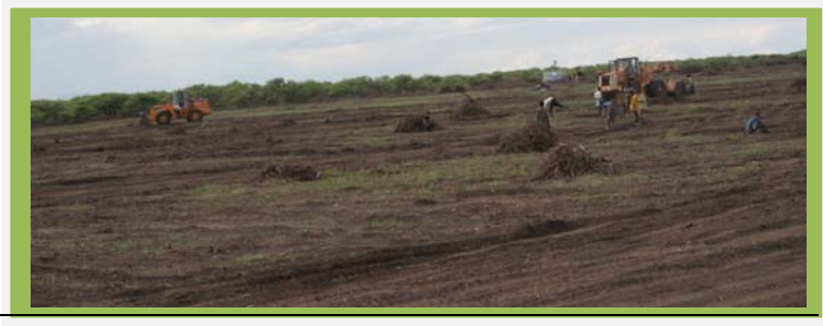
Plate 3: Investment scheme clearing the main elephant ranges on the top of Gobele Valley
